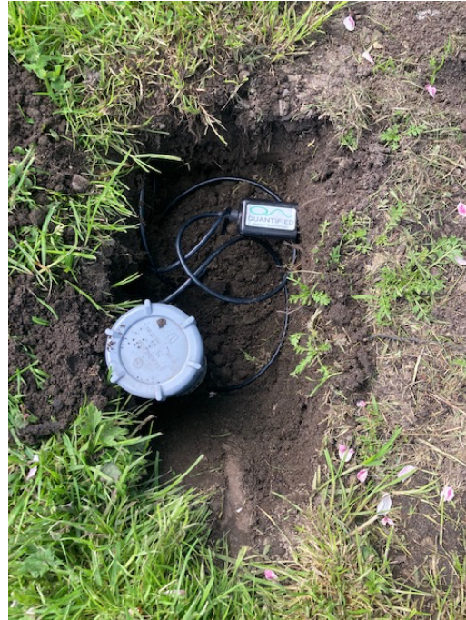
Step 3. Refill the hole to the level where the Poseidon City housing is +/- 2 cm under the top surface.
